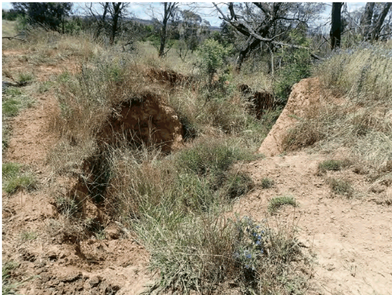
Figure 19 The dam outflow has become eroded as well, indicating that the soils are likely to be highly erosive
